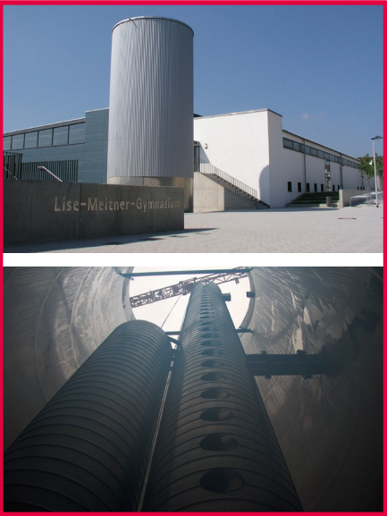
Solar district heating, Crailsheim – Volume: 100 m 3
